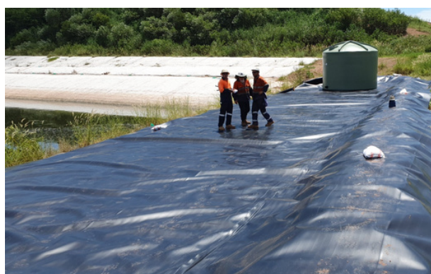
Bunding for treatment plant
