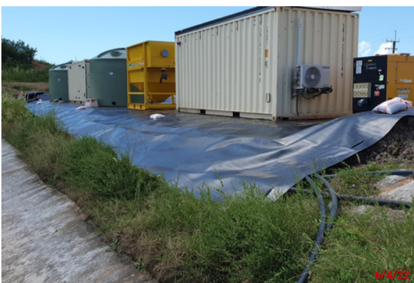
Treatment plant for coagulation, flocculation, breakpoint chlorination, ion exchange, and pH correction.
